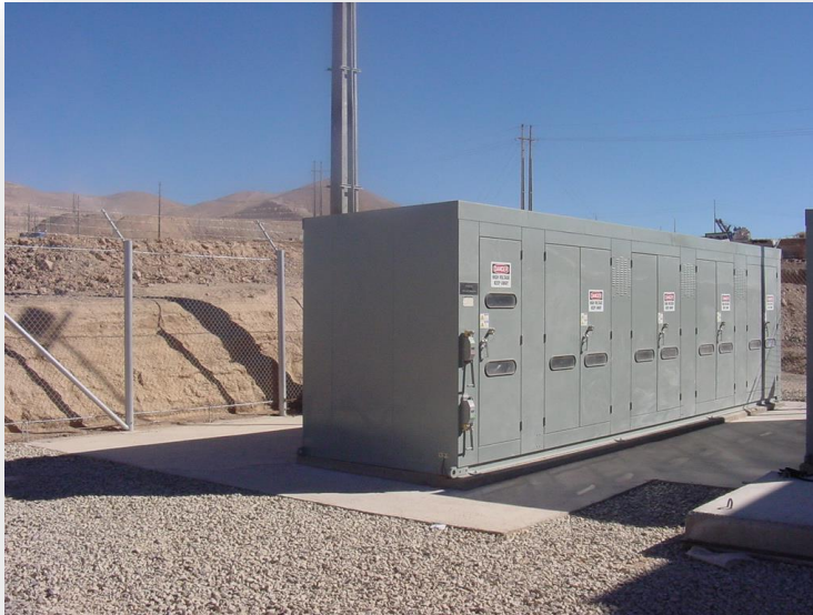
Escondida North, - Bhpbilliton, Chile 9 MVAR+6MVAR, 13.8kV, 150 kV BIL 4-Stage Harmonic Filter System
